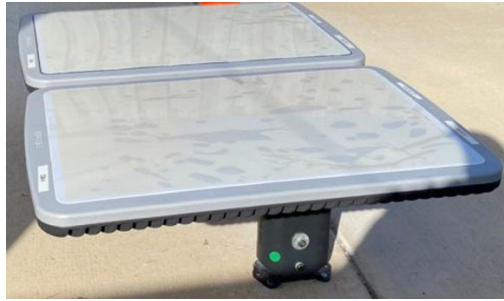
Figure 13: ODU installed with penetrating mount
